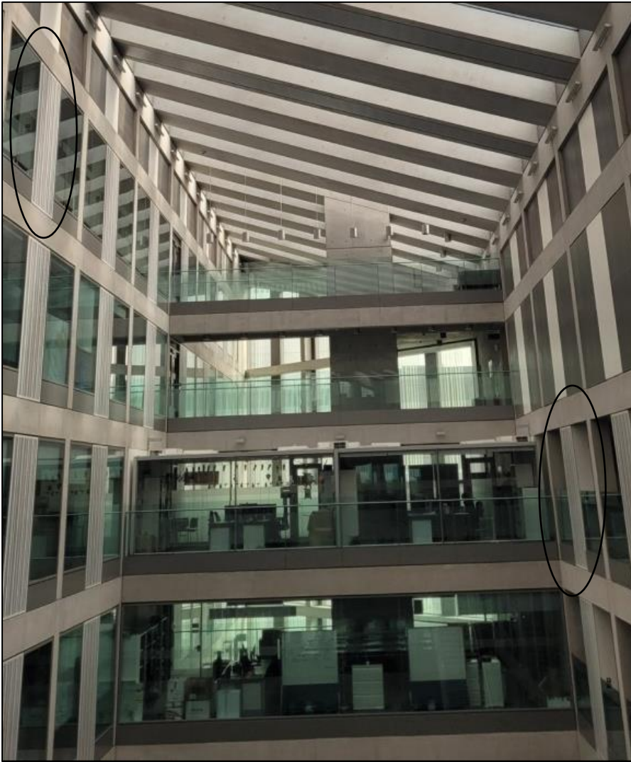
Figure 3.16. The variable-air-volume system vents. They are located on the walls throughout the Business School.
