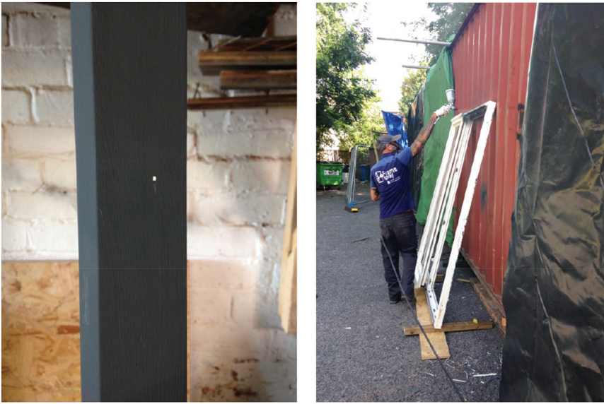
Figure 4. Chipped paint on a window frame from REACH's tests and the application of grey paint using a contractor. (Author's own, 2019).
