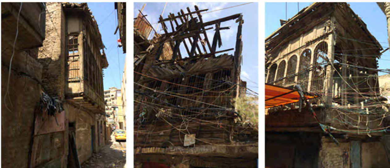
Figure 8. Deterioration of the physical built heritage in Old Rusafa. Source: author’s original images.
