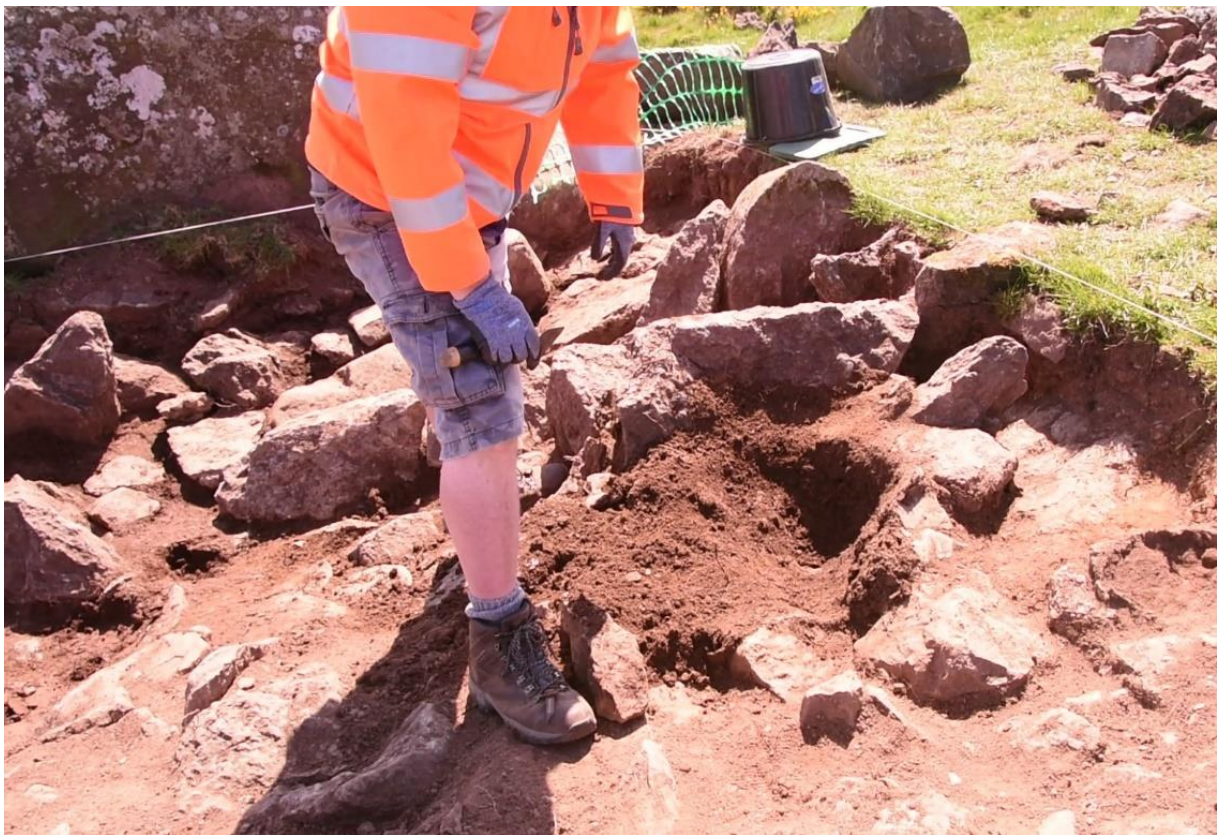
Appendix 29: Still from video showing top of pit of upright stone following its removal.
