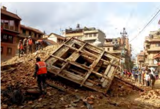
The local people and volunteers aiding the Nepal Army in salvaging and safeguarding the site [Credit: Kai Weise]
