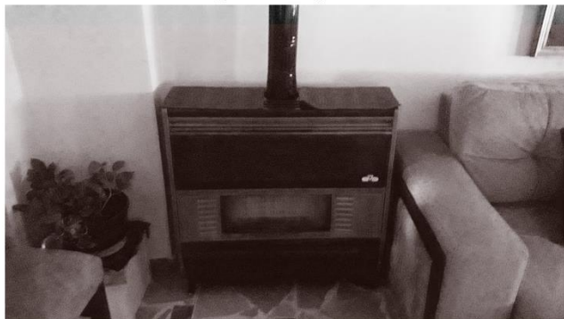
The oil filled heater that is located in the living room.
