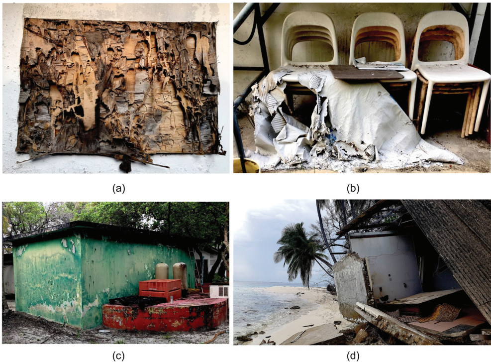
Figure 3. a. Decaying noticeboard (photo by authors) b. Plaster and chairs (source: authors) c. Discoloured green paint (source: authors) d. Destroyed chalet (source: authors).
