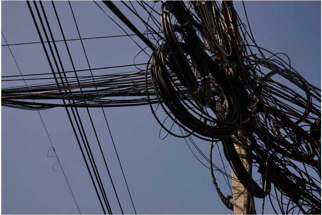
Image 2: Photo of power lines in Bangkok or Manila Prach Gosavitra © 2019
