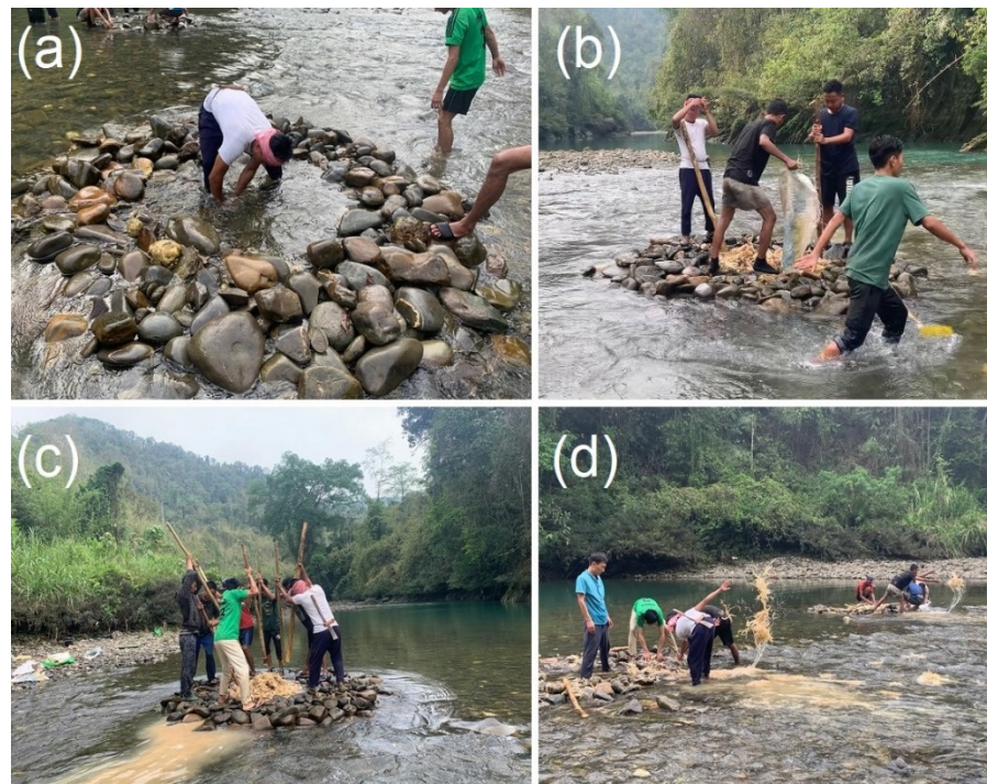
Figure 8. (a) Construction of stone platform for pounding and threshing of roots, (b) transfer of the roots of D. elliptica for pounding, (c) pounding of D. elliptica showing the release of yellowish extracts from the roots and (d) releasing the pounded root into the river current, during intra-tribal community fishing practices in Nagaland, Northeast India.
