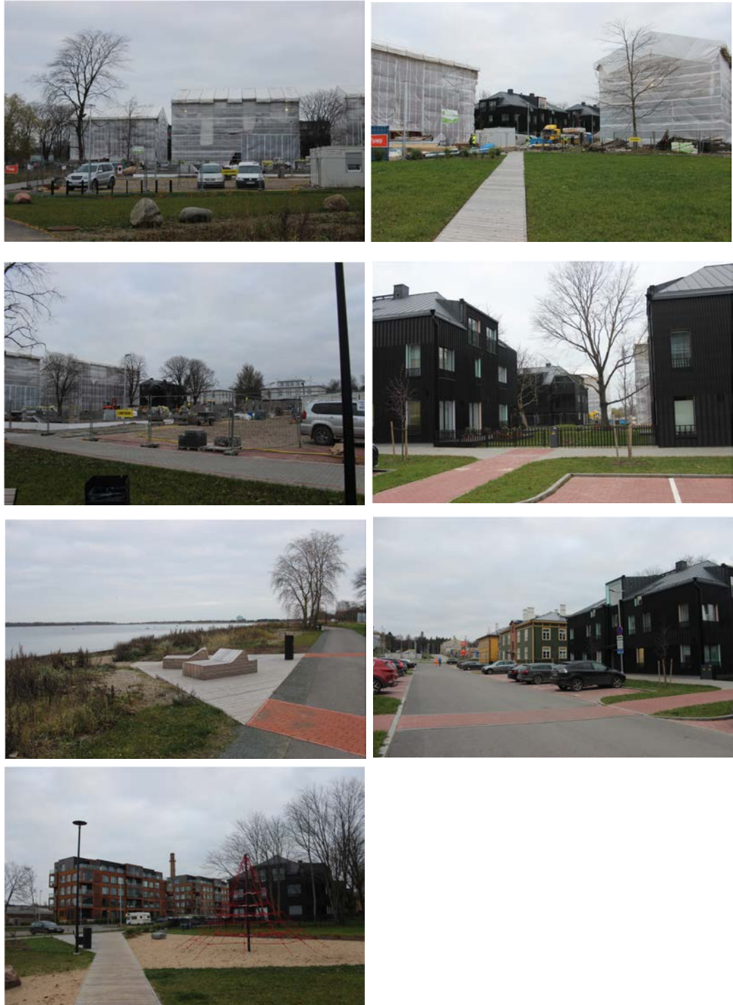
Figures 457–463: The lower lines are starting to take the shape of a functioning neighbourhood. This is supported by nearly finished landscaping surrounding the buildings. Works are underway on some of the timber buildings that will be restored (Source: Kurik, 2020)
