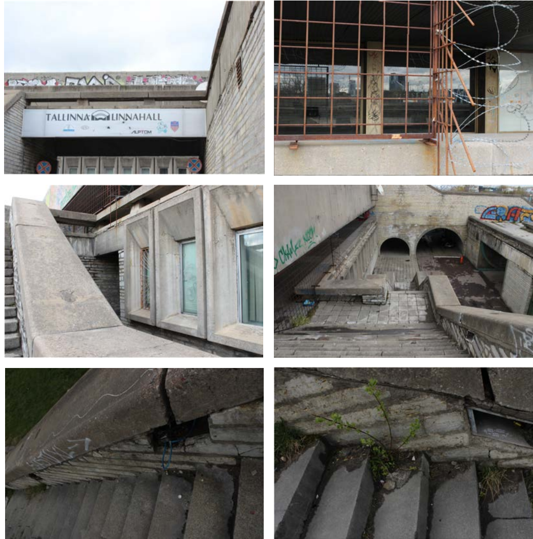
Figures 105–110: The building is showing signs of deterioration, but predominantly a lack of maintenance. This is evident from weeds growing through the structure, loose wires and uncovered electrics, but also loose slates (Source: Kurik, 2014)
