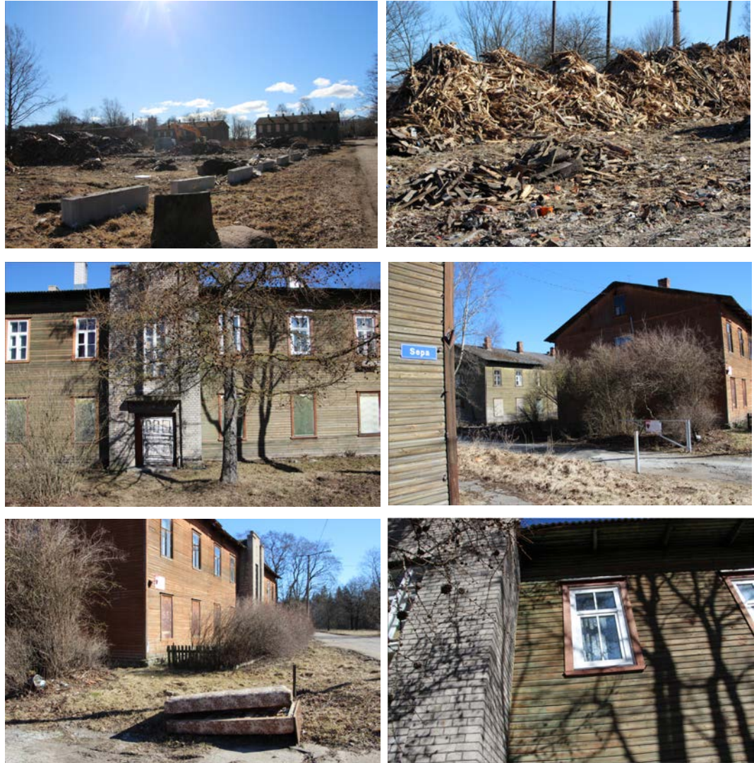
Figures 384–389: Demolition has started on the upper lines. The leftover timber has been gathered in huge piles and diggers are working. I note what seem to be recently installed PVC windows on one of the buildings (Source: Kurik, 2017)
