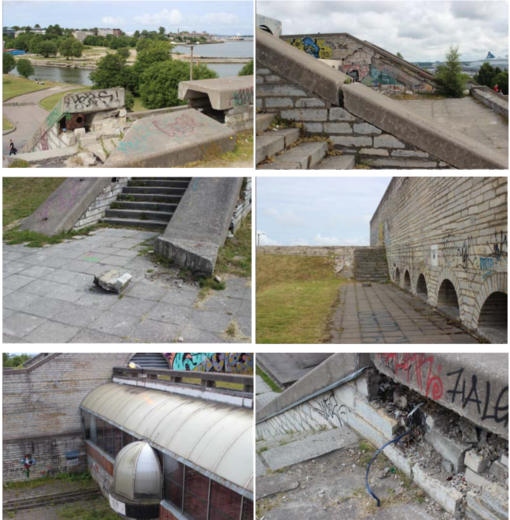
Figures 165–170: Looking closely at the building's condition it seems like parts of it are sliding – gravity is pulling the decorative slate and concrete layers off the structure and revealing a messy skeleton. From a distance, this architectural landmark looks intact, but a closer look reveals a site that has been left to nature (Source: Kurik, 2017).
