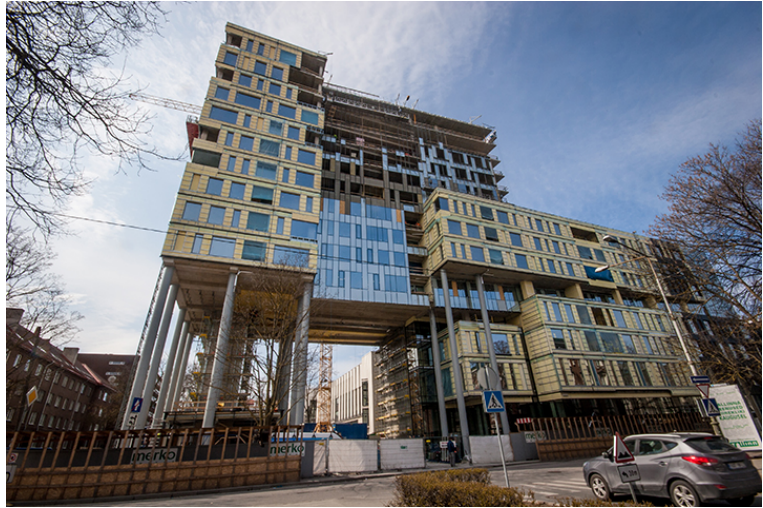
Figure 14: A building on Rävåla Avenue designed to accommodate a never realised urban vision (Source: Maran, 2014: online)
