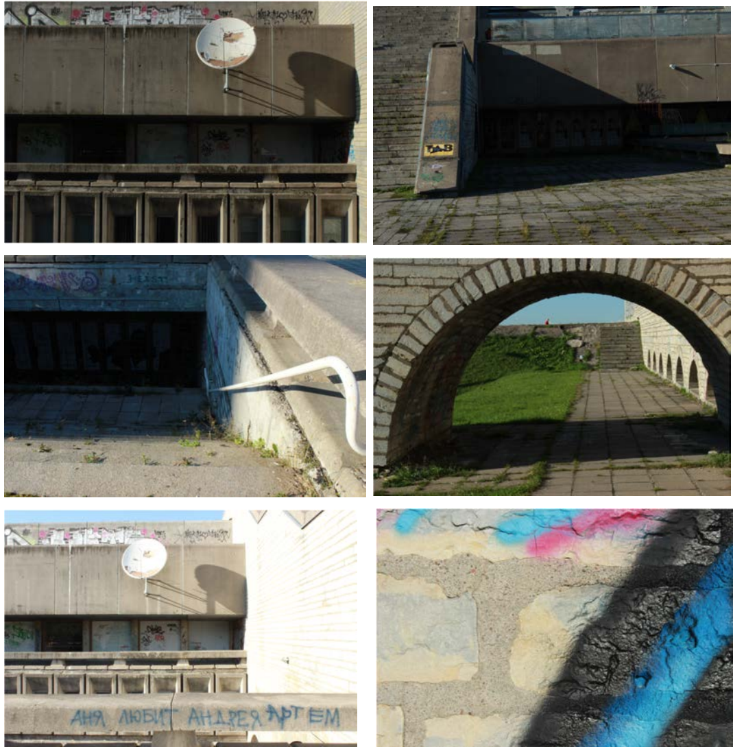
Figures 91–96: The walls of Linnahall function as a canvas for social commentary and seemingly neutral colourful scribbles (Source: Kurik, 2013)
