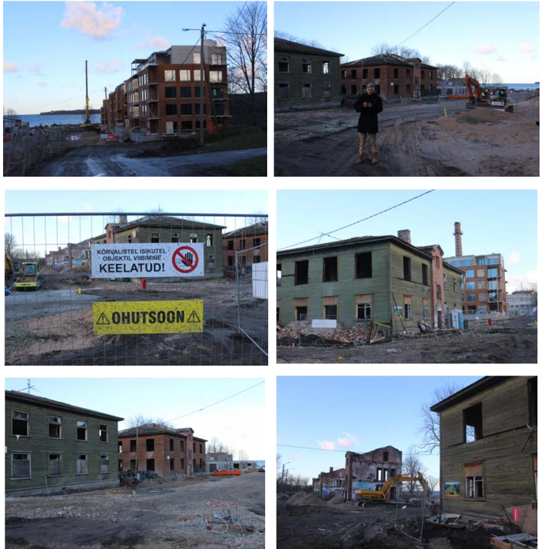
Figures 415–420: Works have started on the lower lines – the first phase of redevelopment. Historic buildings that will be restored have been gutted and will be brought back into use with different floor plans. A new taller apartment building is also in its final stages of development (Source: Kurik, 2018)
