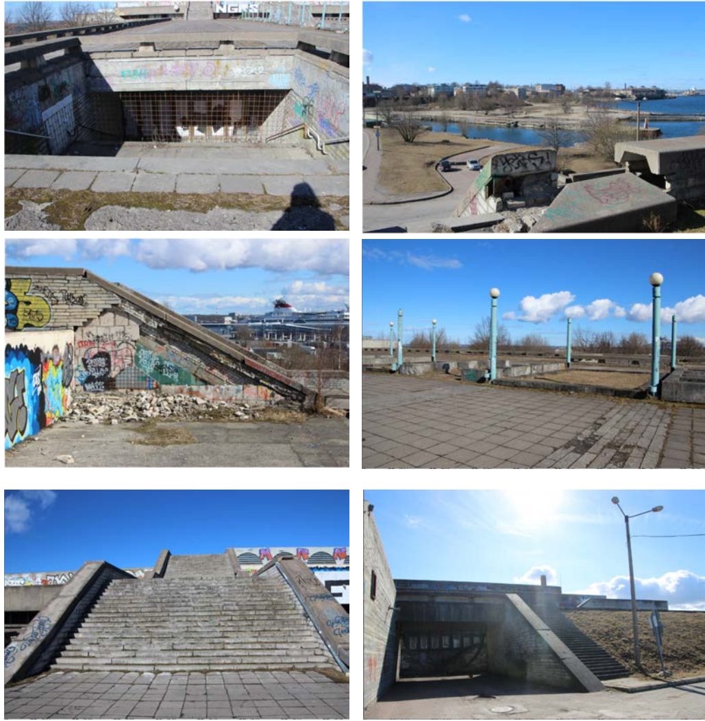
Figures 145-150: During this site visit the building seemed especially abandoned as the rooftop was empty – it has become typical to see it in use as a public space. The deteriorating 'facade' of the concert hall revealed the poor quality construction that the architect of the building has made reference to. Layers of slate have peeled off to reveal a structure that has been built from a mismatch of materials (Source: Kurik, 2017).
