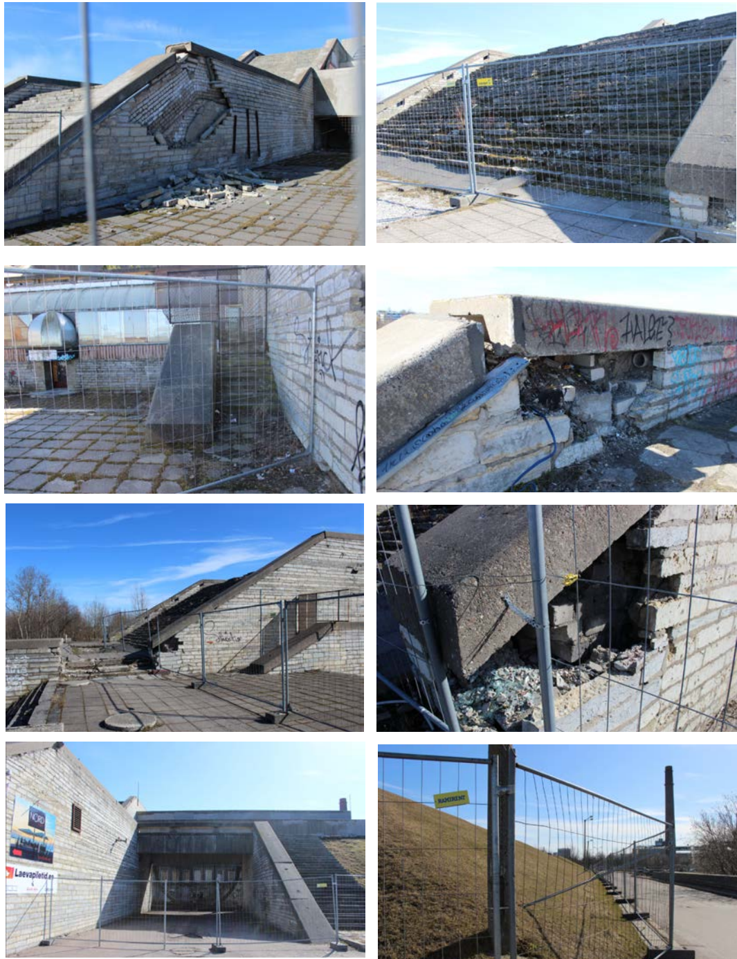
Figures 205–212: Fencing demonstrating the poor condition of the building. The central promenade running across the building is still accessible, but it is no longer possible to explore the curious pathways characteristic to the building (Source: Kurik, 2019).
