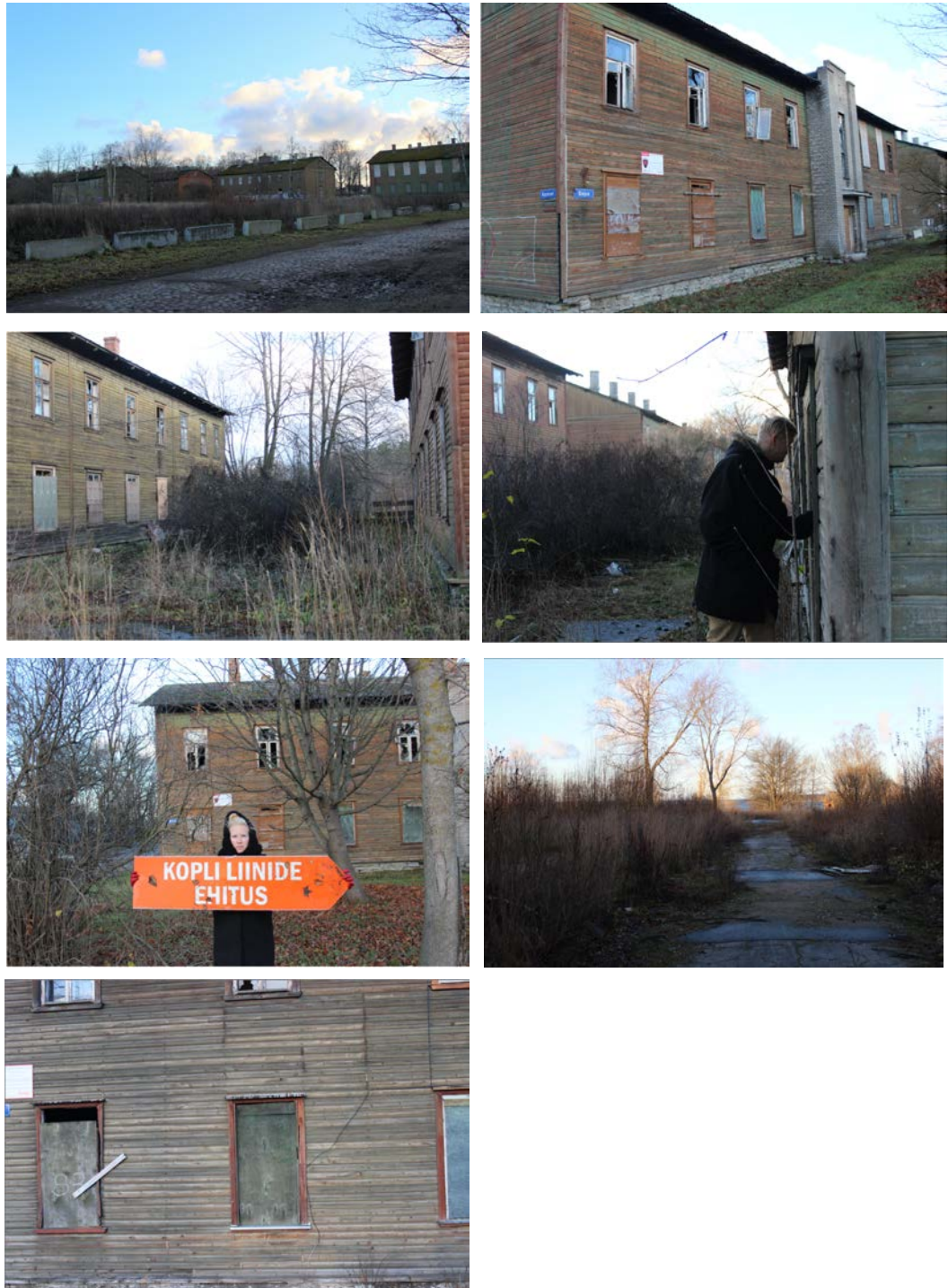
Figures 402–408: The upper lines are designated to be the final stage of the redevelopment. In their present state they have been cleaned and left waiting for a new future. The ground floor windows of buildings have been boarded, but the upper floors remain exposed to the elements. It
