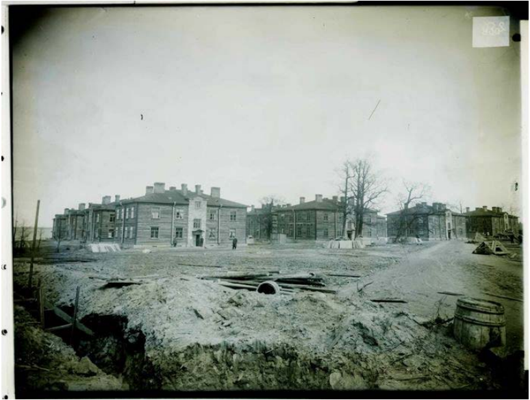
Figure 310: The construction of residential buildings on lower lines, 1910. First phase of housing that was most likely completed by 1914 (Source: Fotis, 1910: online)
