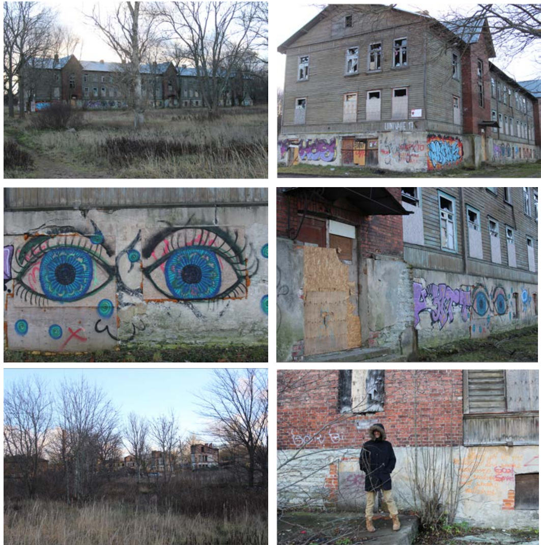
Figures 409–414: There are further signs of deterioration on the central lines, including broken windows on upper floors leaving the building exposed. It is also evident that there are still informal uses in the building (Source: Kurik, 2018)
