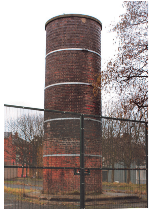
Figure 10: Ventilation shaft for the Victoria tunnel, Shenstone Street.
