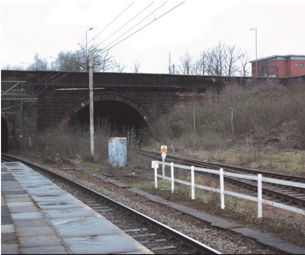
Figure 7: The Victoria tunnel portal on the right with one to Lime Street on the left, Edge Hill Station.
