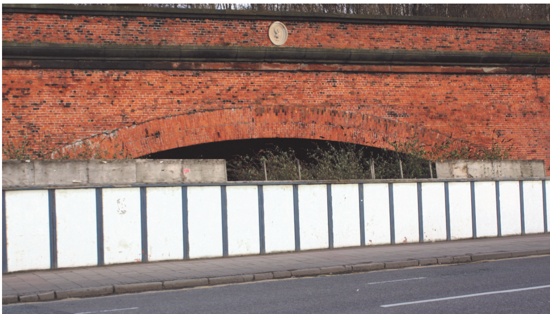
Figure 16: Railway bridge built by the L & YR to span the Waterloo tunnel (1849), Great Howard Street.
