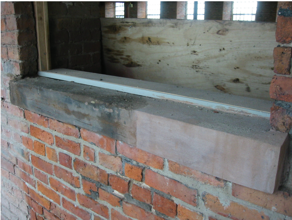
Figure 2. Isolated sandstone repair at Murrays Mills, Manchester. A restoration approach? Image courtesy of Jonathan Davis. All rights reserved.
