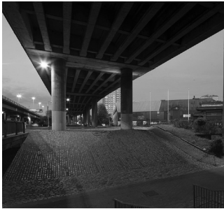
Fig. 4. Underpass built as envisioned in 1965 concept sketches without the footfall and connectivity, Glasgow, 5 December 2017.
