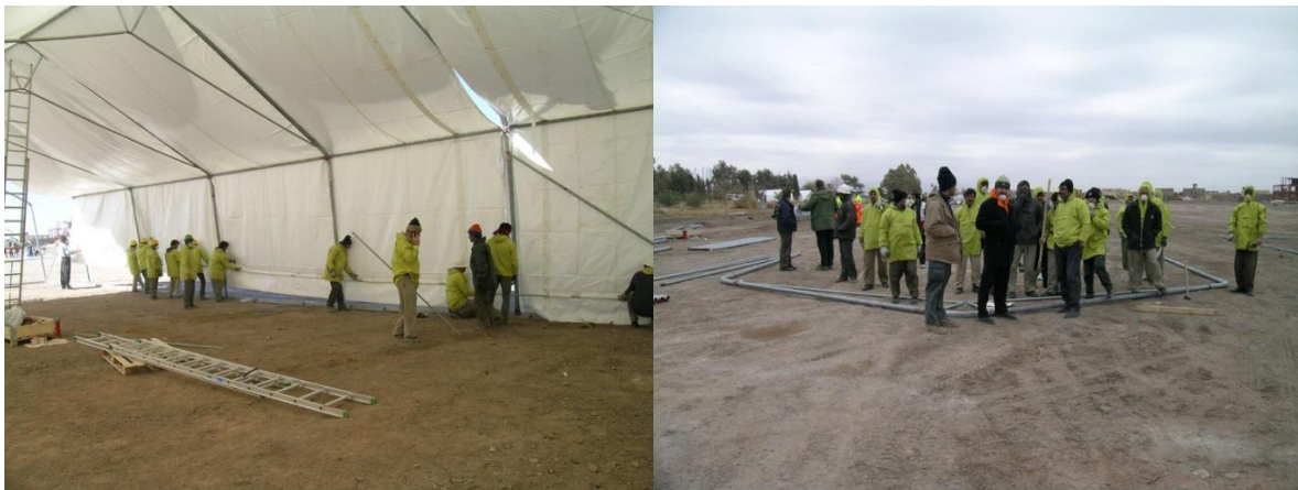
Figure 4.6: Emergency NGOs erecting large-scale tents in the Bam post-earthquake scenario, Amir Camp (By author)
