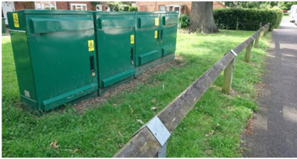
Fig. 1 ESMU with one PEU (on the right) and two ESUs (on the left) installed on a grass verge near a footpath in residential area in Bracknell, UK
