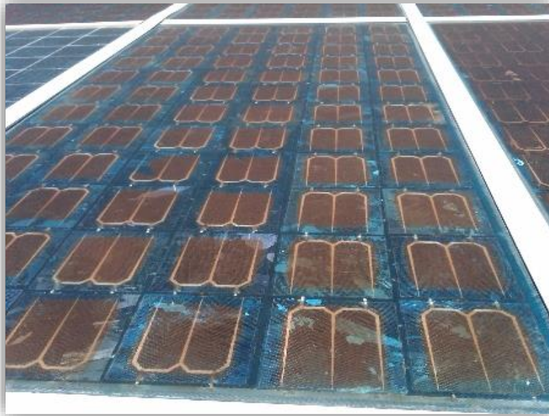
Figure 2-2 Photo of 20 year old photovoltaic panels that suffer from discoloration due to exposure to high humidity and changing temperature outdoor environment in Mexico [17, 18].
