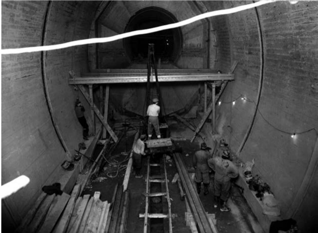
Figure 8. Original photograph documenting the construction of the GUTE , dated March 1956. The scale of the main equipment tunnel is evident and this was eventually subdivided to create two working levels. The formwork for concreting in the main tunnels was steel, but the connecting points between the tunnels were made by specialist joiners from timber. (Source: Photograph by tunnel engineer Patrick Gough. Courtesy of George Coney.)
